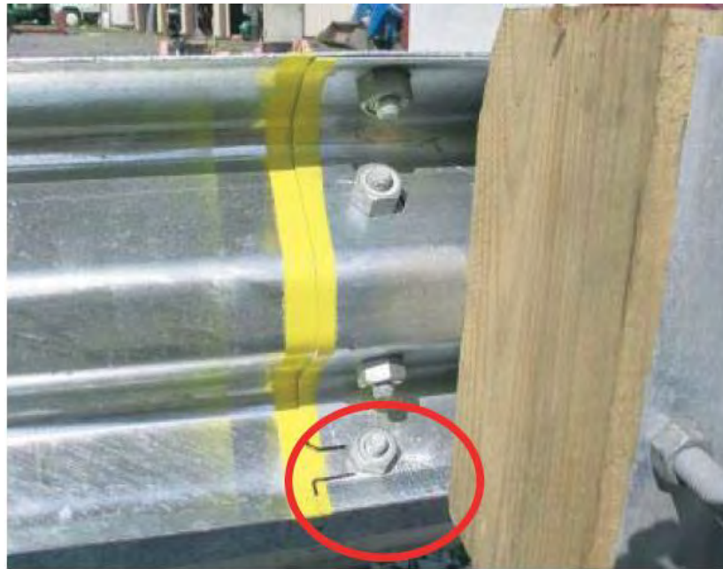
Figure 49. Fabricated splice damage mode evaluated by Gabler et al. [Gabler10]
