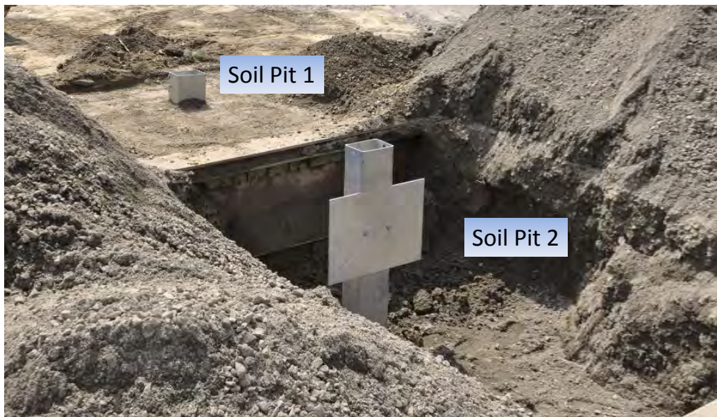
Figure 289. Photograph of anchor tubes with soil plates during installation (from preliminary Test 14011B).
