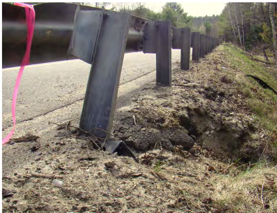
Figure 244. Example of soil erosion at a guardrail post.
