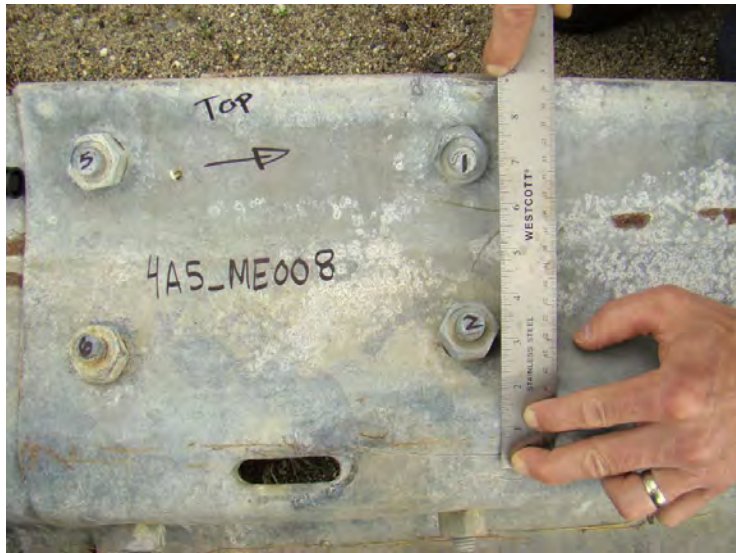
Figure 325. Rail flattening – Rail flattening and rail crush at each quadrant of the splice is measured from the center of the w-beam to the top/bottom edge at the splice bolts.
