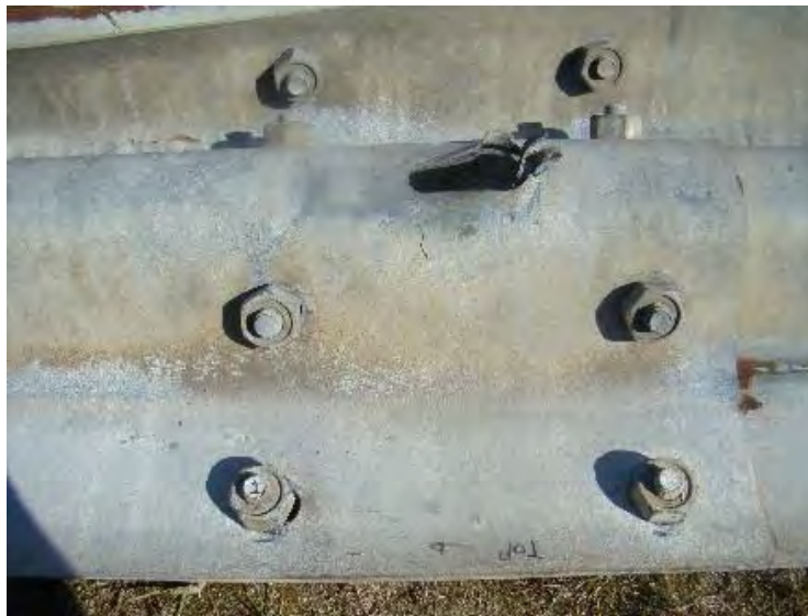
Figure 330. Horizontal tear in post bolt hole – This photo shows evidence of both stretching and a horizontal tear in the post bolt hole.
