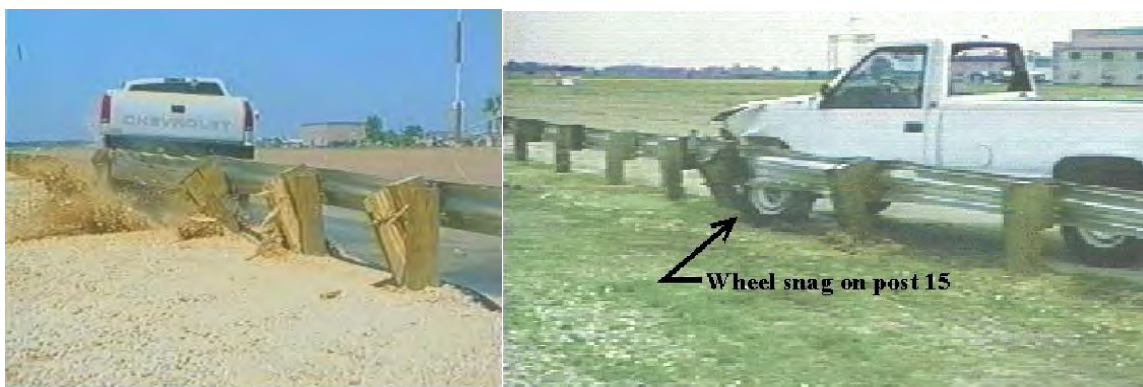
Figure 59. Typical damage modes for wood post guardrails.[Bullard00;Mak95]
