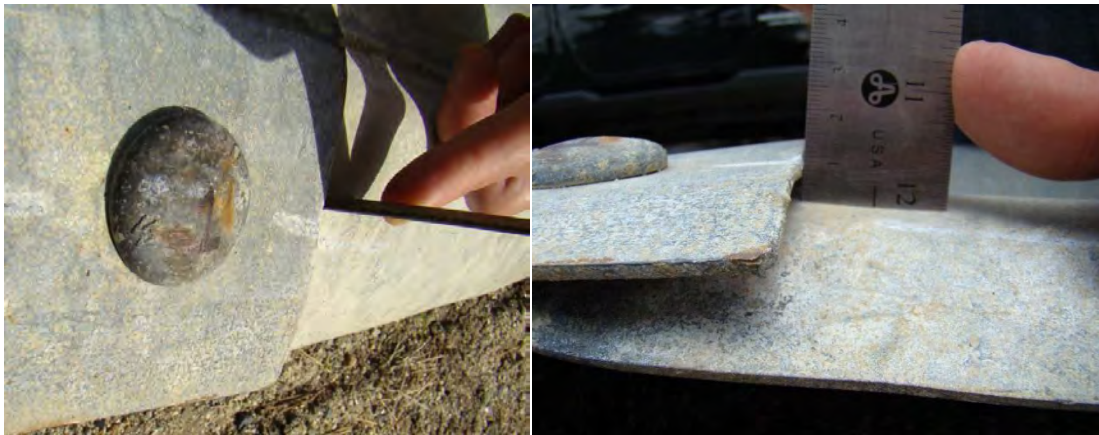
Figure 326. Rail separation - Lateral gap between rail elements at splice connection (measurements taken at locations adjacent to the eight splice bolts).
