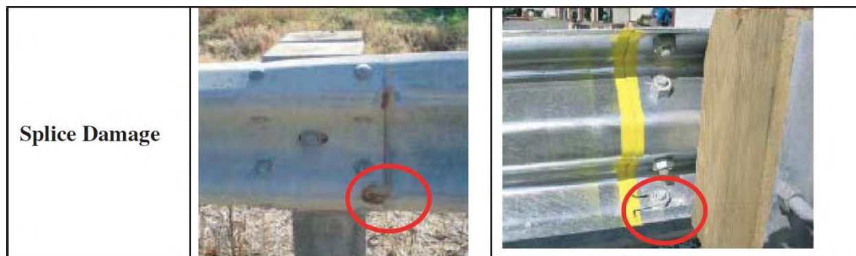
(a) Field Installation damage
