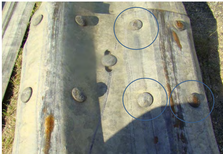
Figure 328. Gouging – Gouging of splice-bolts into w-beam panel is evidenced by rotation of the bolt about the vertical axis.
