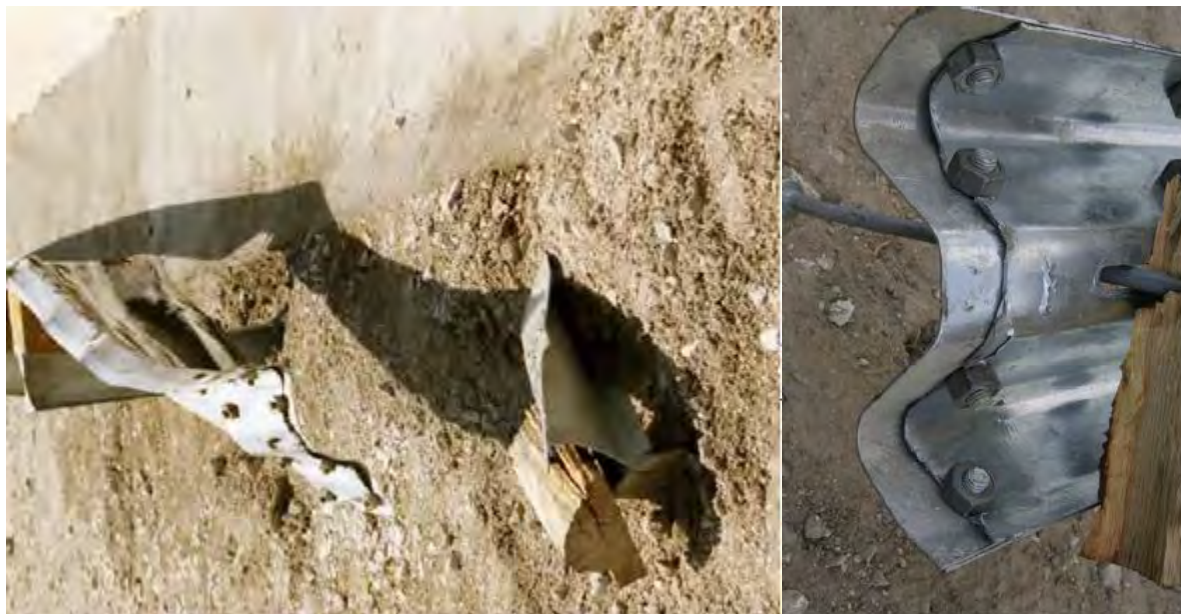
Figure 65. Blockout split during Test NEC-1 (left) and in Test 405160-1-1 (right). [Polivka00a; Buth06]
