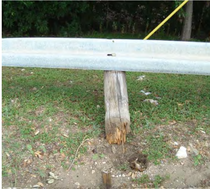
Figure 63. Post fracture below groundline due to rot. [Photo provided by Mark Bloshock]
