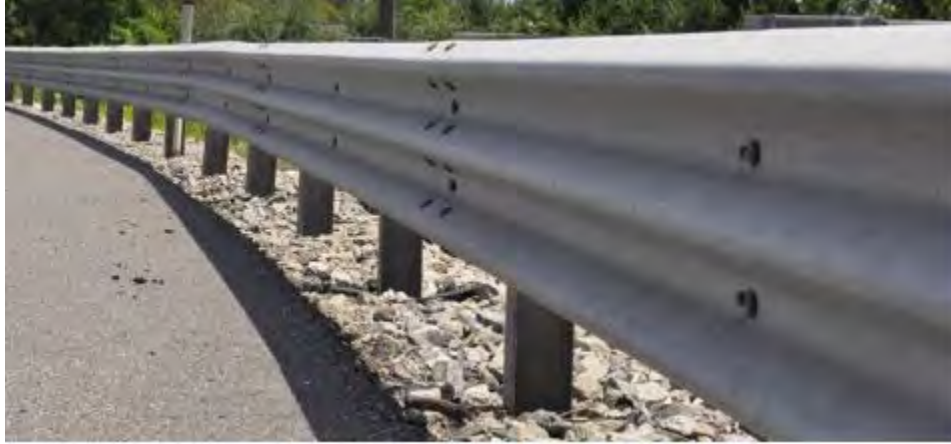
Figure 69. Photo of the standard thrie-beam guardrail.
