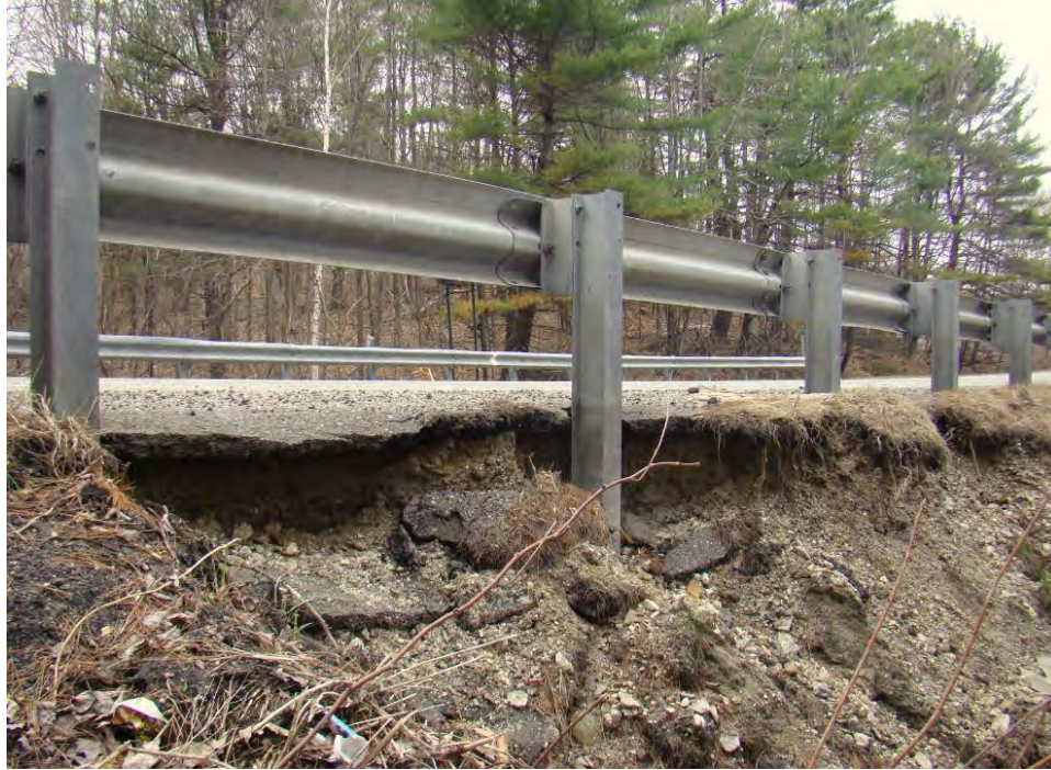
Figure 245. Example of severe soil erosion at multiple posts.
