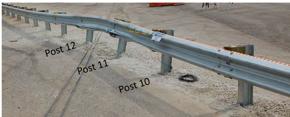
Figure 217. Damage to guardrail in low-speed impact test C08C3-027-1. [Fleck08a]
