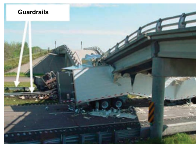
(b) Superstructure was not continuous, and the pier system was not redundant.
