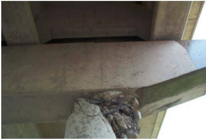
Column-cap connection failure
