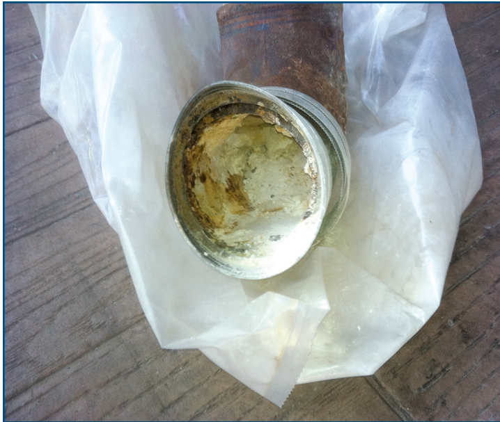
Figure 7 – Drain line plugged with fireproofing.
